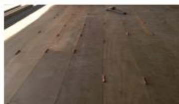
1MM SPACES PULLED OUT WITHIN 24 HOURS
