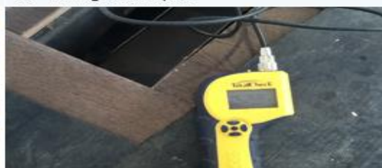
Moisture meter- Floor Board testing at 11.1% (only 2% variation is acceptable between sub floor and floor board)
