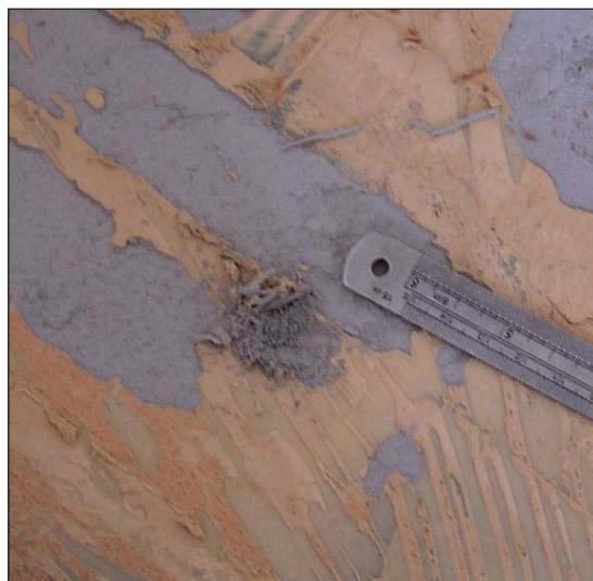
Leveling compound with insufficient strength
